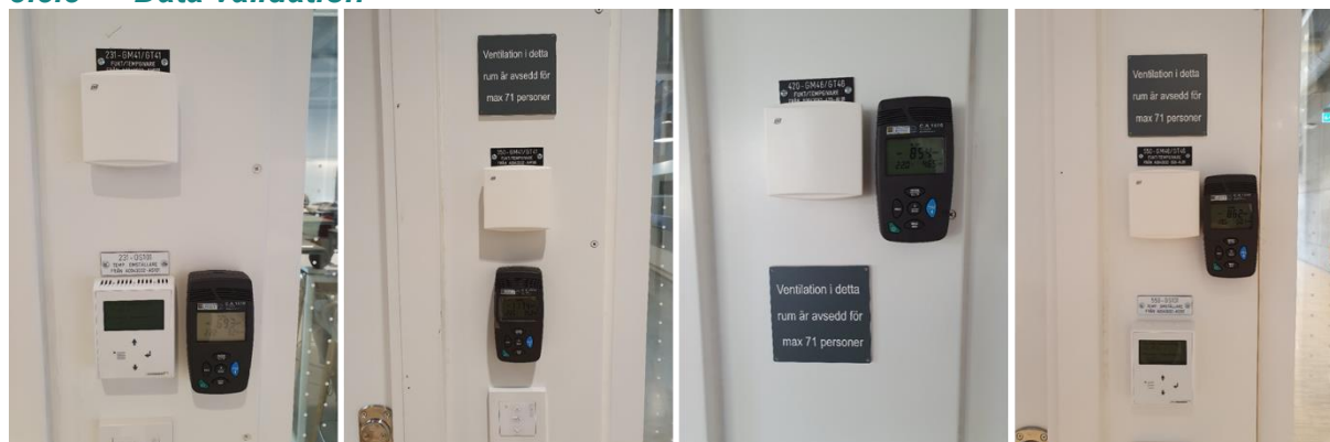
Figure 60 Device Chauvin-Arnoux CA1510 installed in the classrooms of Testbed AH during a data validation campaign.
